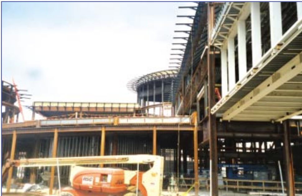
Abraham Lincoln Presidential Museum, Springfield, Illinois Client: United Steel Fabricators, Inc., Indianapolis, Indiana
