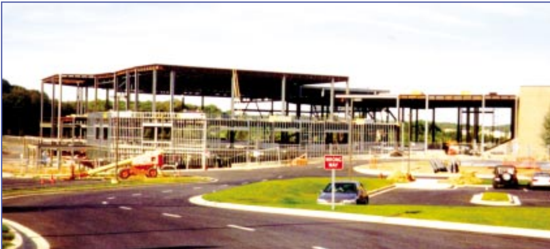
Covenant Life Church, Gaithersburg, MD Client: Structural Steel Fabricators, Linthicum Heights, MD
